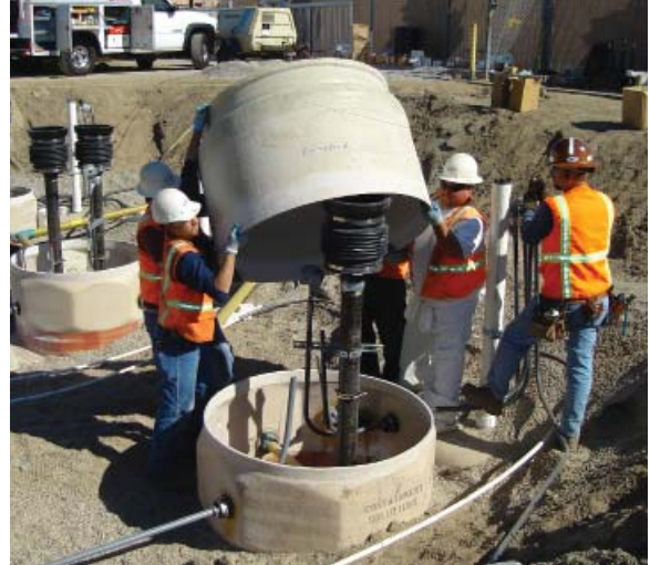
Fiberglass tank sumps are installed to protect the surrounding environment from potential leaks and provide a watertight access point to service pumps and piping.
